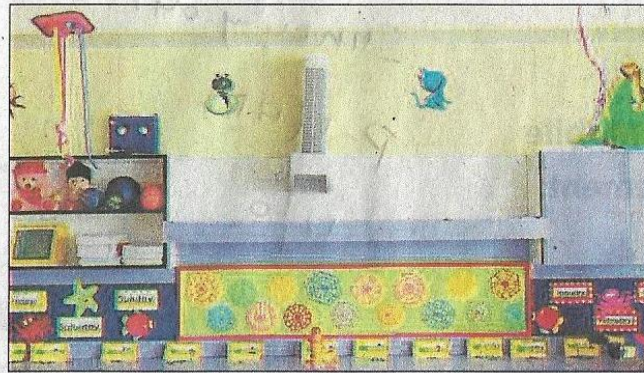
■ The air purifier installed at Suncity School.
